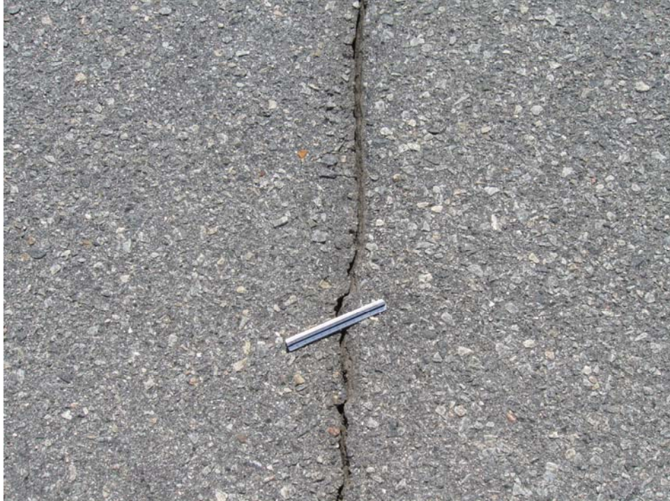
TAMGRA-10. Longitudinal and Transverse Cracking (Sample Unit #24).
