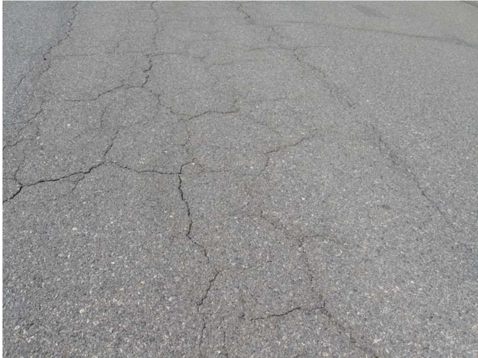
TAMGRA-10. Block Cracking (Sample Unit #21).
