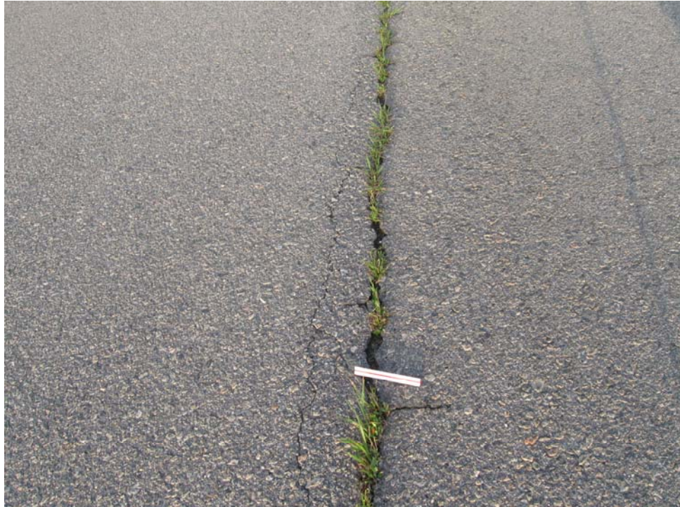
A01MGRA-10. Longitudinal and Transverse Cracking (Sample Unit #26).
