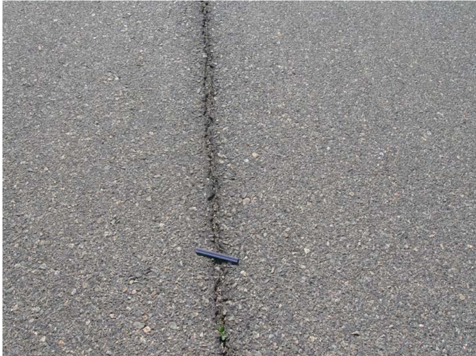
TCMGRA-20. Longitudinal and Transverse Cracking (Sample Unit #70).
