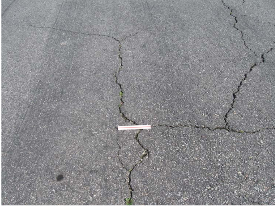
A01MGRA-80. Longitudinal and Transverse Cracking (Sample Unit #13).
