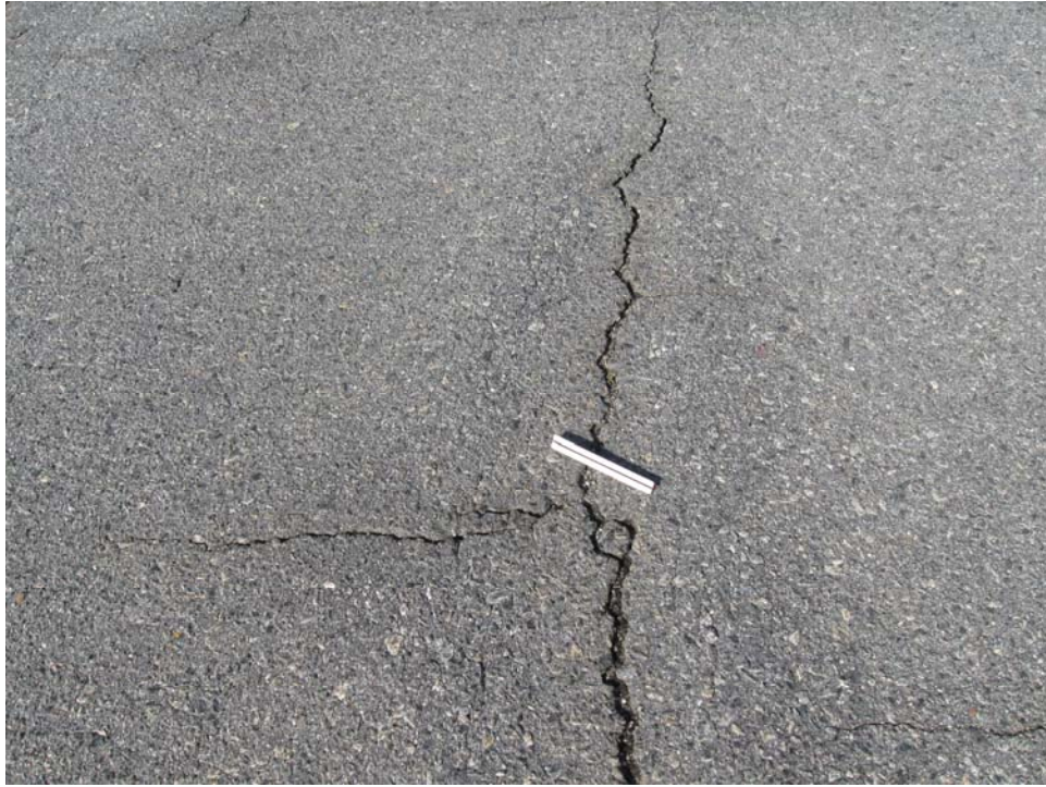
A01MGRA-70. Longitudinal and Transverse Cracking (Sample Unit #08).
