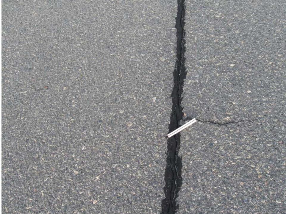
A01MGRA-20. Longitudinal and Transverse Cracking (Sample Unit #41).
