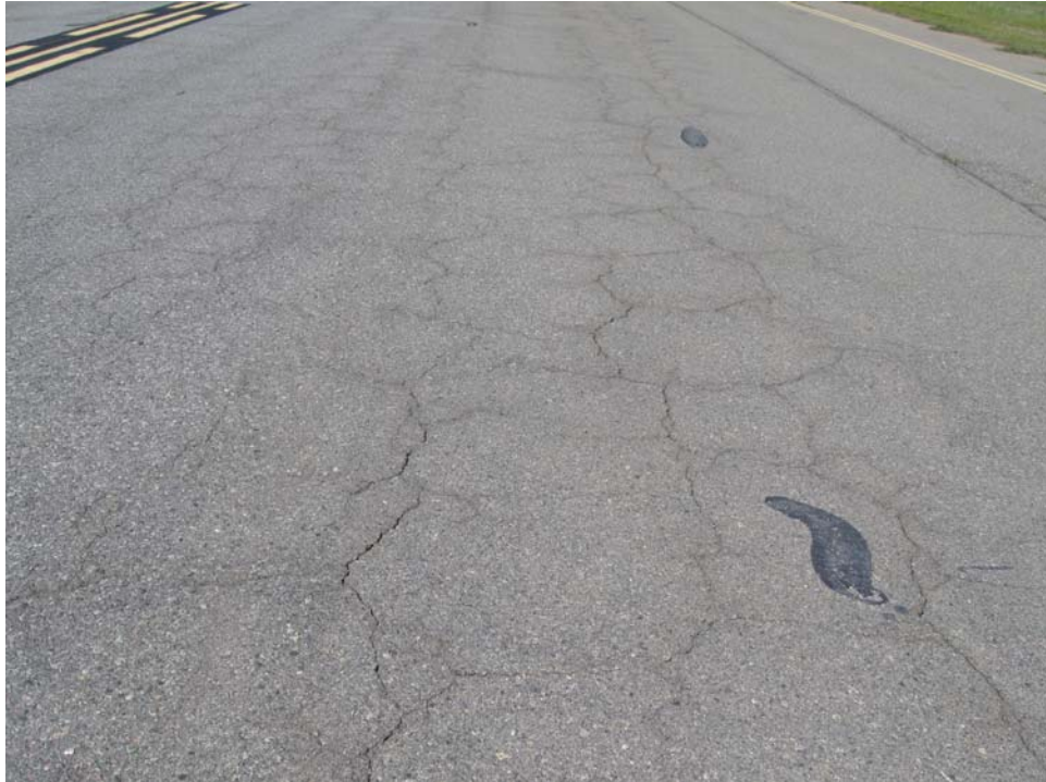
TCMGRA-10. Block Cracking (Sample Unit #14).
