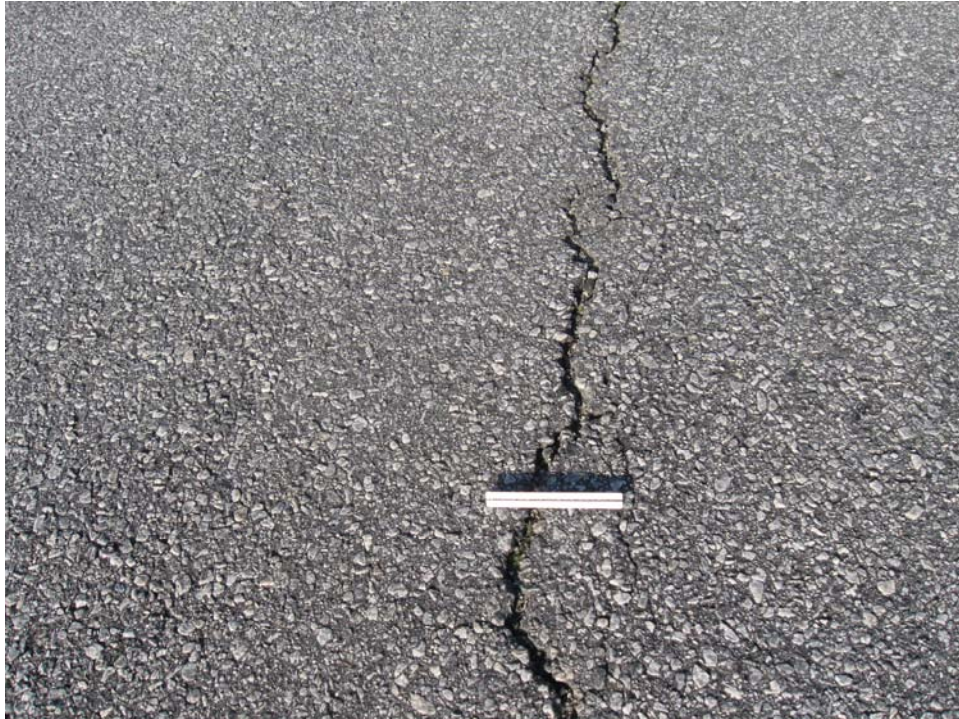
A01MGRA-50. Longitudinal and Transverse Cracking (Sample Unit #16).
