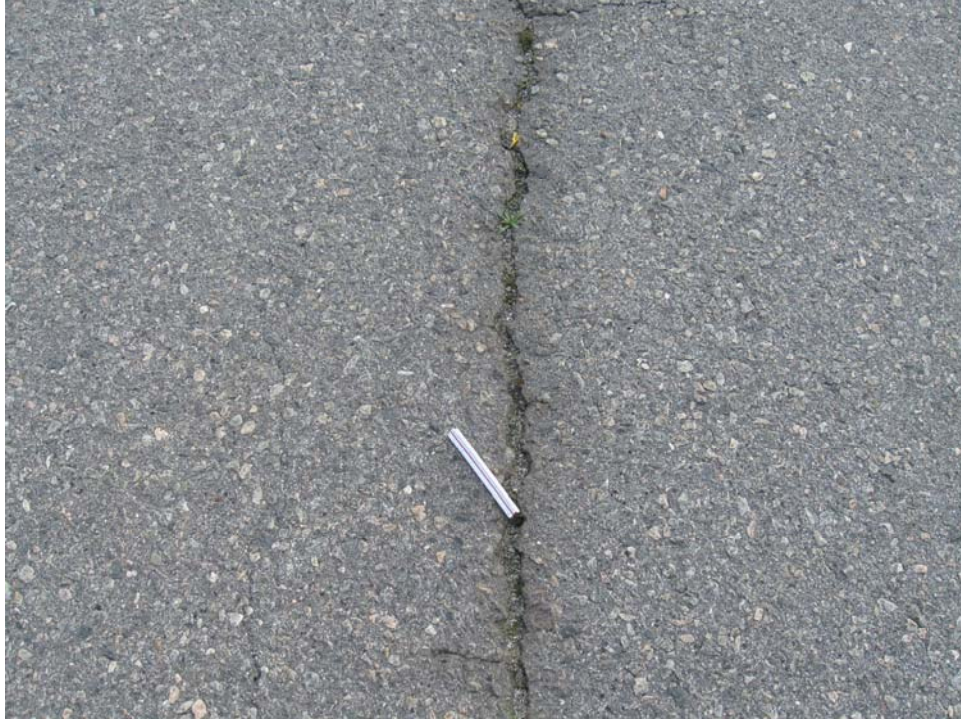
TB3MGRA-10. Longitudinal and Transverse Cracking (Sample Unit #04).
