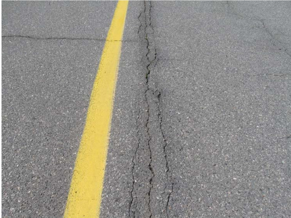
TAMGRA-10. Longitudinal and Transverse Cracking (Sample Unit #30).
