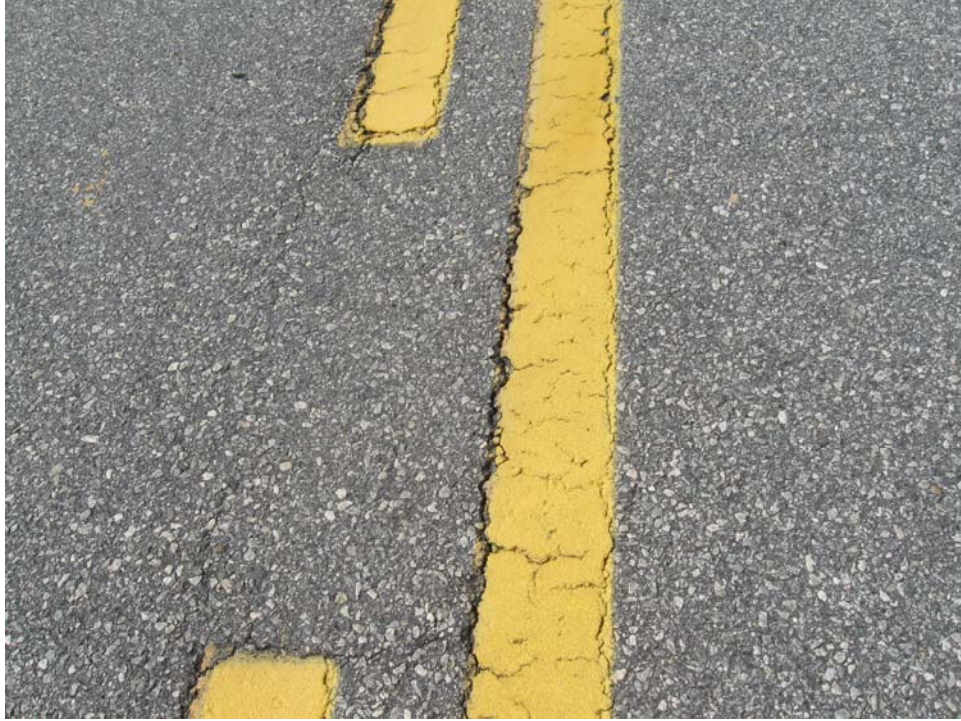
A01MGRA-40. Unsatisfactory Paint.
