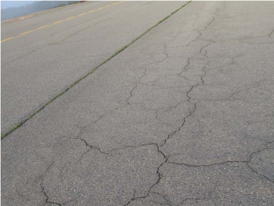
A01MGRA-10. Block Cracking (Sample Unit #26).
