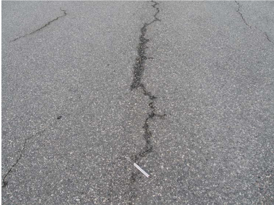
A01MGRA-30. Longitudinal and Transverse Cracking (Sample Unit #01).
