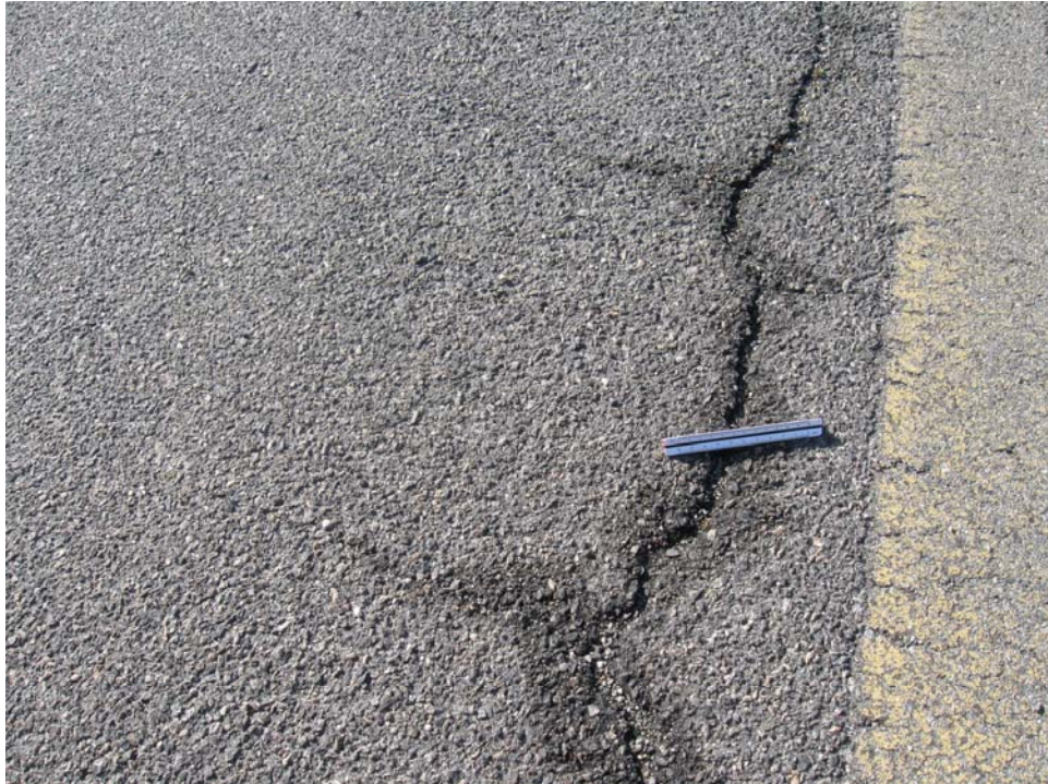
A01MGRA-60. Longitudinal and Transverse Cracking (Sample Unit #03).
