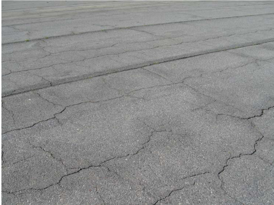
A01MGRA-70. Block Cracking (Sample Unit #08).
