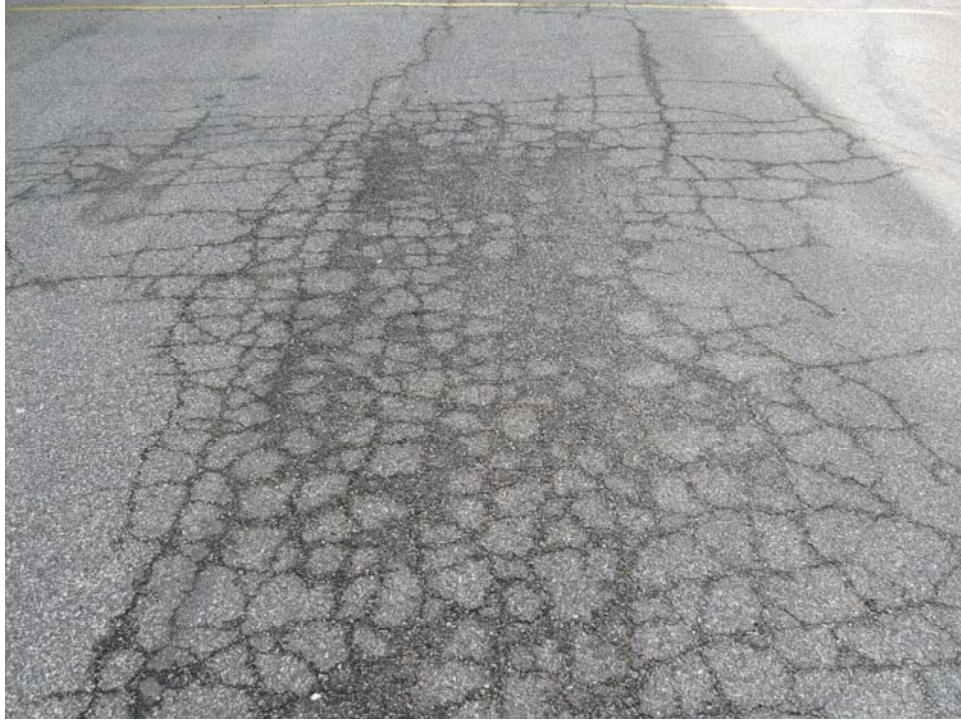
TGAMGRA-10. Alligator Cracking (Sample Unit #07).
