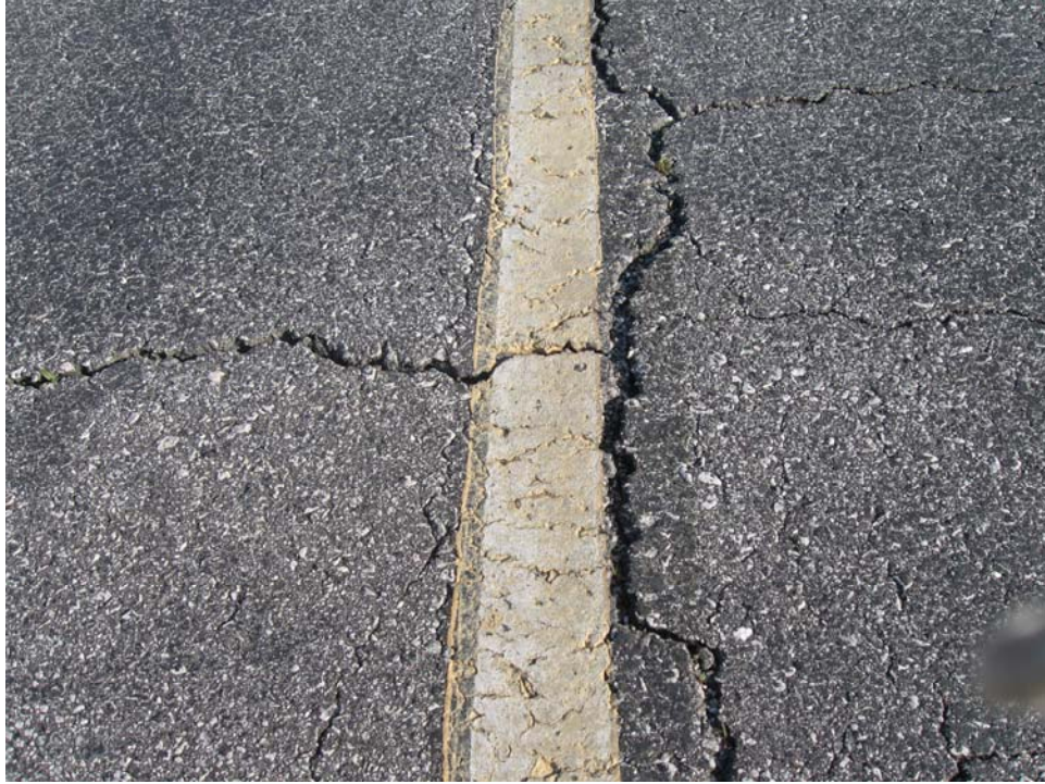
A01MGRA-50. Unsatisfactory Paint.
