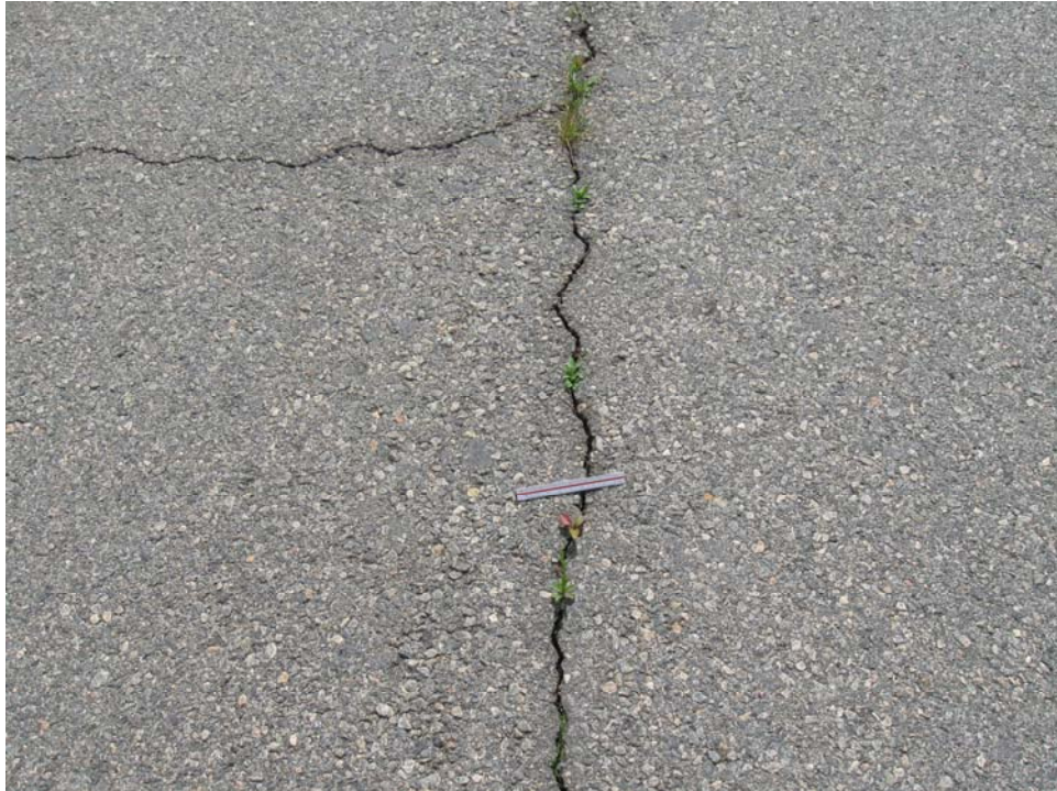
TGAMGRA-10. Longitudinal and Transverse Cracking (Sample Unit #11).
