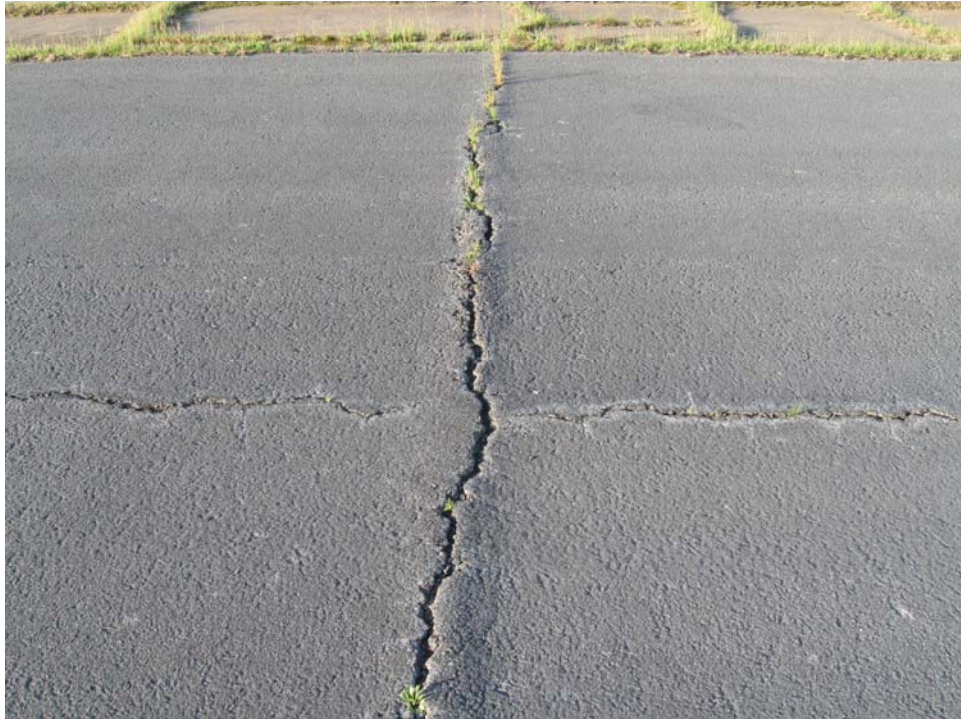
R1311MGRA-10S. Longitudinal and Transverse Cracking (Sample Unit #03).
