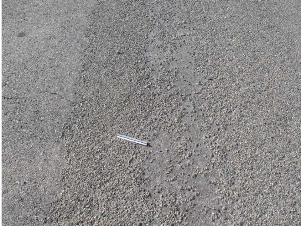
A01MGRA-60. Raveling (Sample Unit #03).
