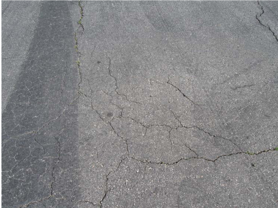
A01MGRA-80. Alligator Cracking (Sample Unit #13).
