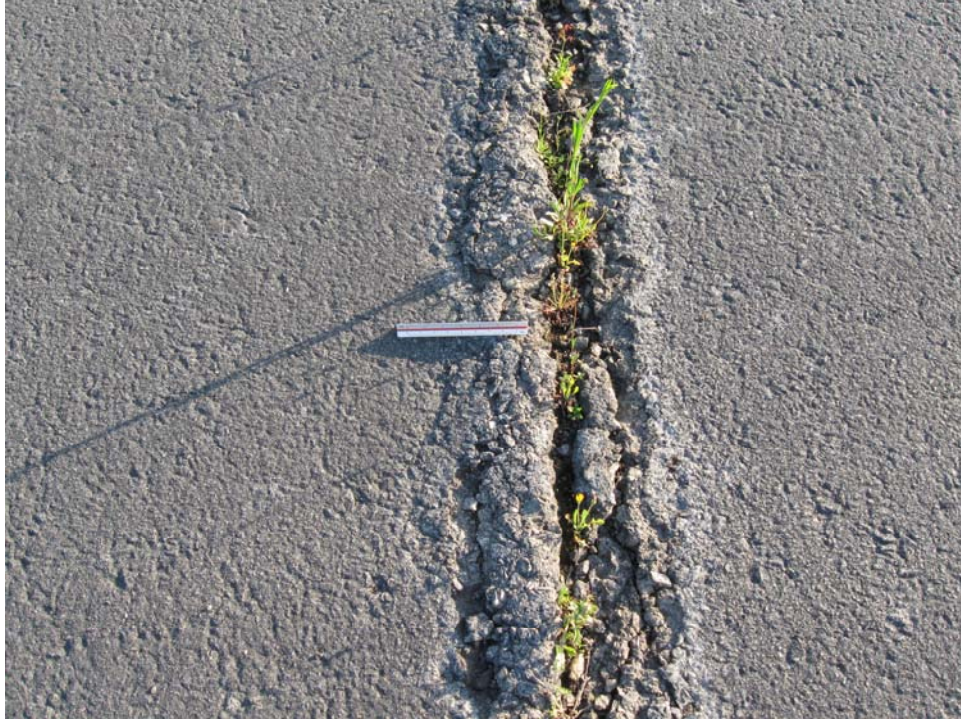
R1311MGRA-10N. Longitudinal and Transverse Cracking (Sample Unit #02).
