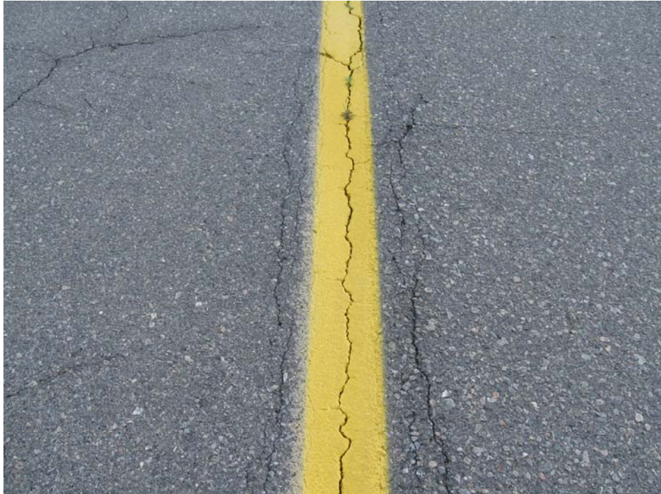
TB3MGRA-10. Satisfactory Paint.
