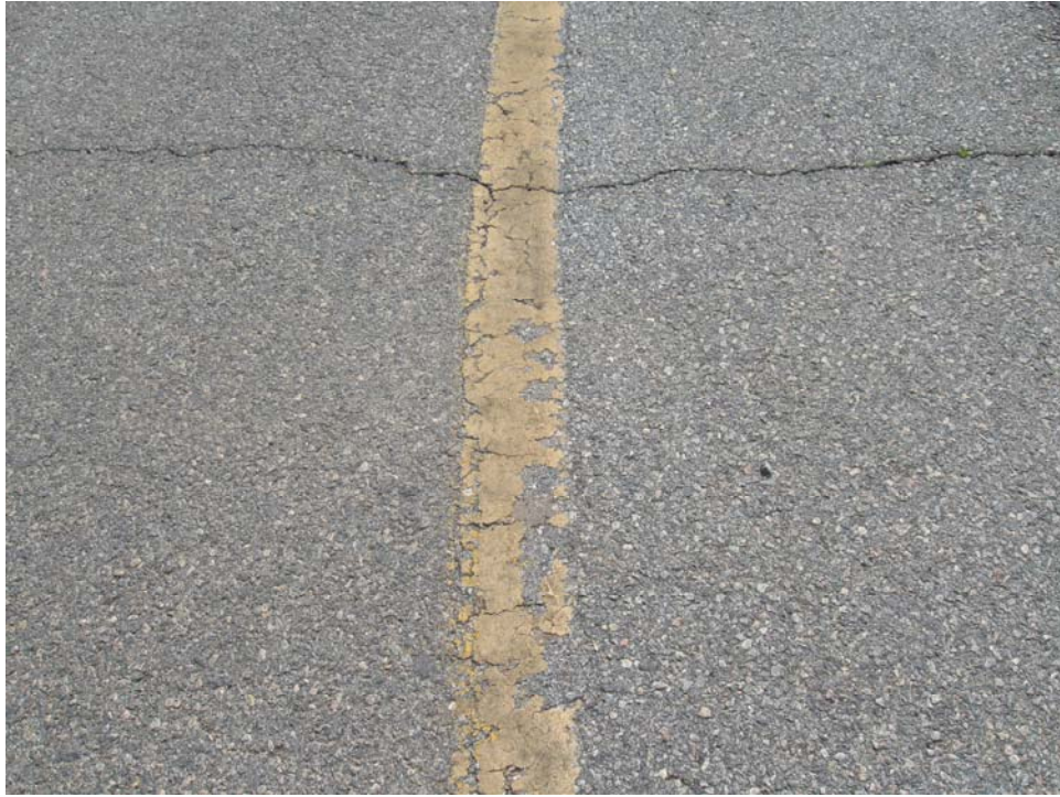
TGAMGRA-10. Unsatisfactory Paint.
