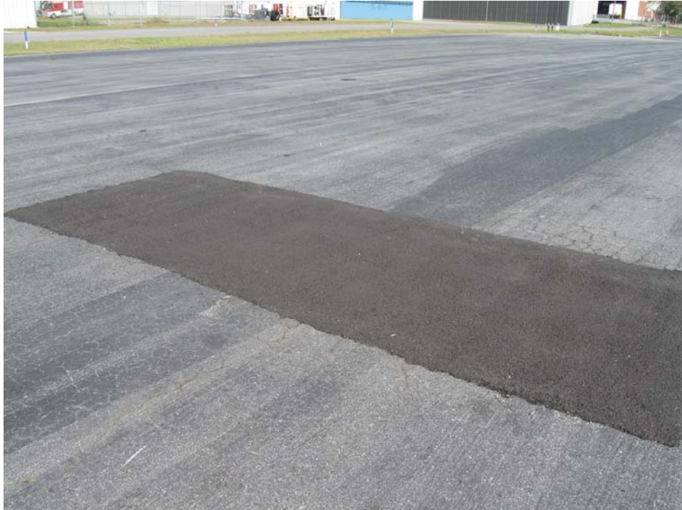
A01MGRA-80. Patching (Sample Unit #13).
