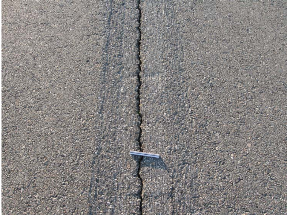
R1311MGRA-10C. Longitudinal and Transverse Cracking (Sample Unit #08).
