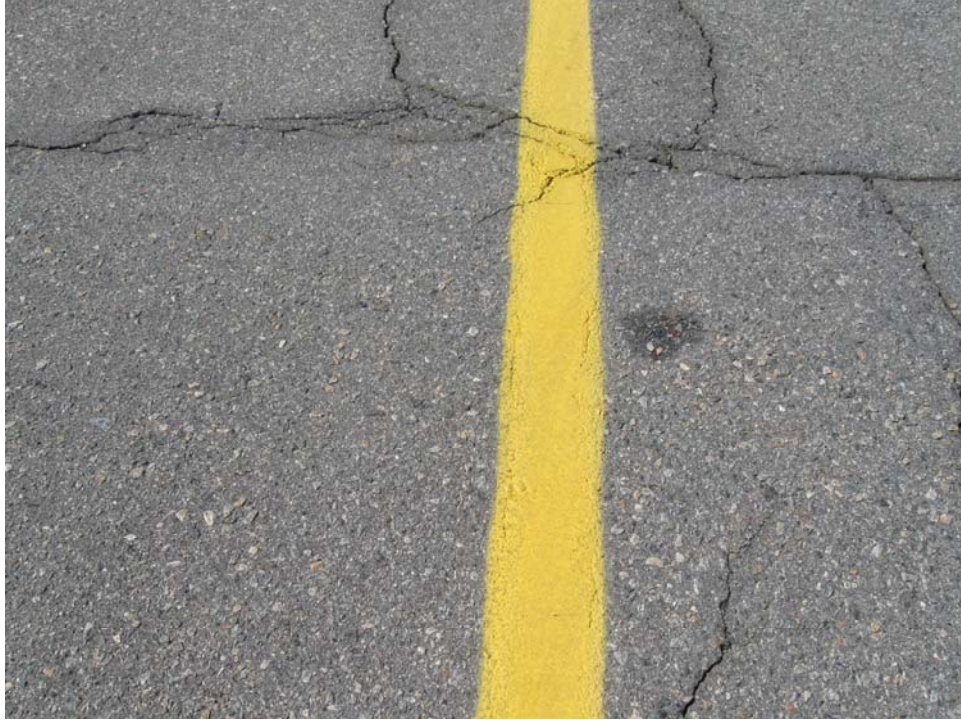
TAMGRA-10. Satisfactory Paint.
