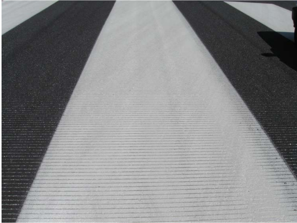
R523MGRA-10N. Satisfactory Paint.
