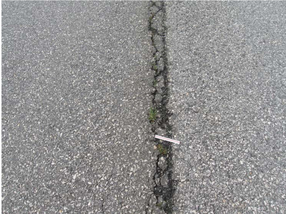
A01MGRA-40. Longitudinal and Transverse Cracking (Sample Unit #14).
