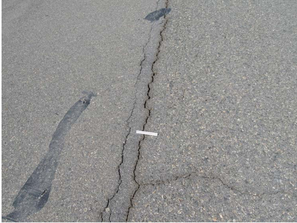
TCMGRA-10. Longitudinal and Transverse Cracking (Sample Unit #14).
