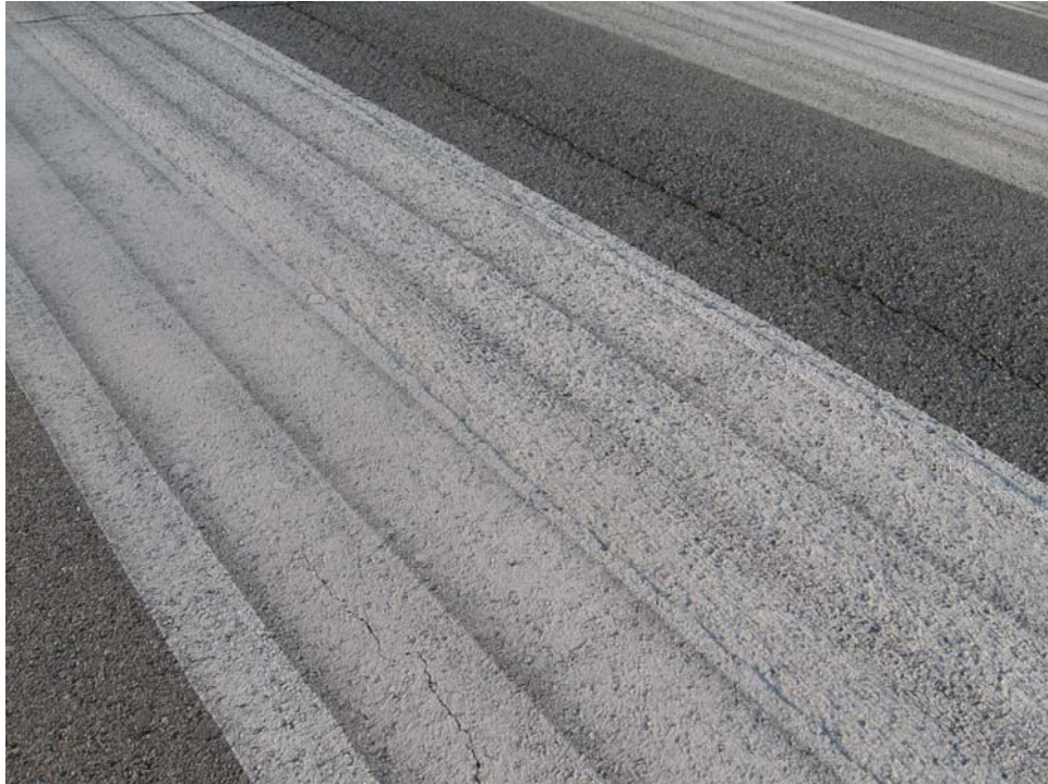
R1311MGRA-10C. Unsatisfactory Paint.
