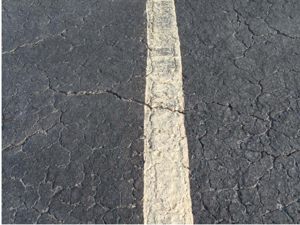
A01MGRA-20. Unsatisfactory Paint.
