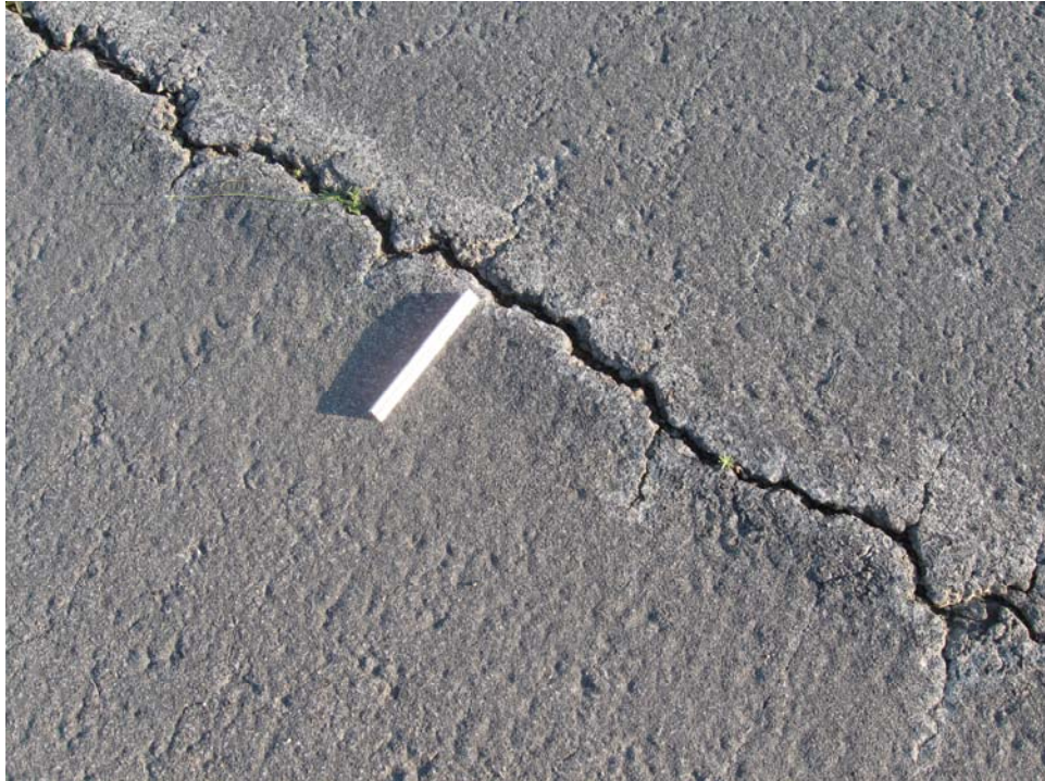
R1311MGRA-10N. Longitudinal and Transverse Cracking (Sample Unit #02) (2).
